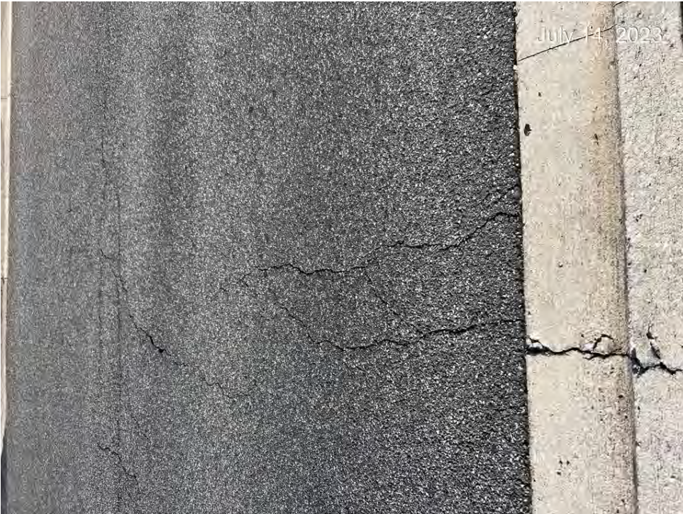
Broken curb and crack asphalt at settled area.
