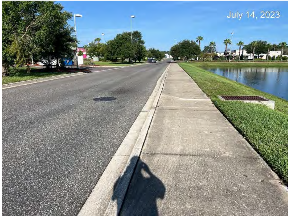
Settling at downstream storm manhole.
