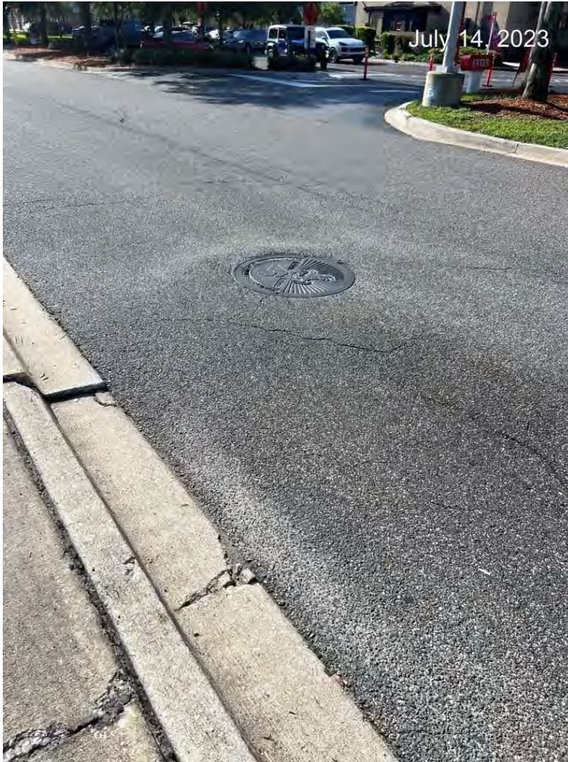
Evidence of settling at the control structure and curbing.
